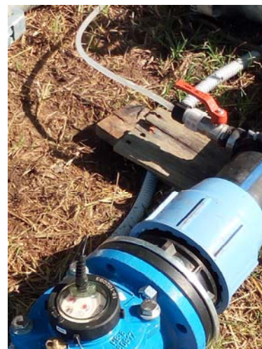
Injection point and meter
