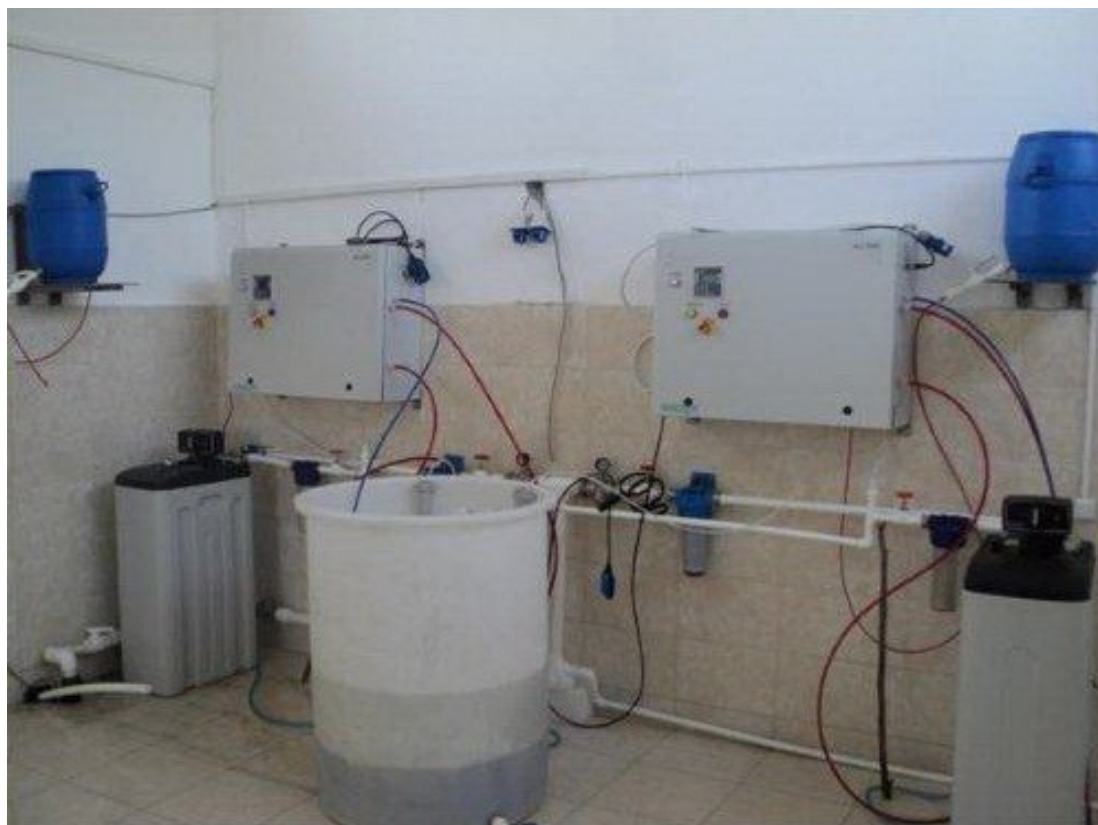
ELA-2000s with brine tanks, water softeners and anolyte tank
