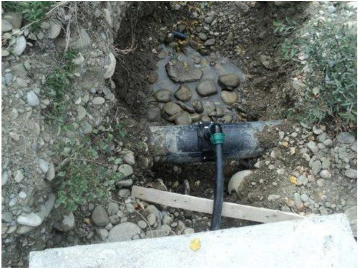
Anolyte injection point
