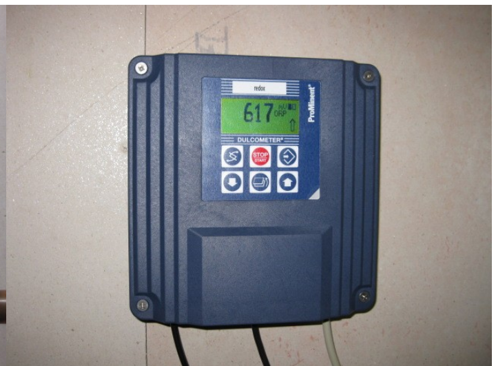
Redox control unit
