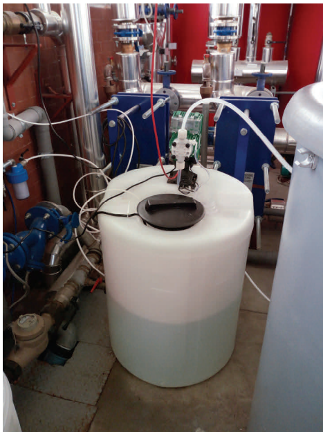
Dosing station on main water
