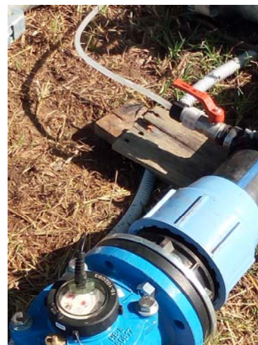
Injection point and meter
