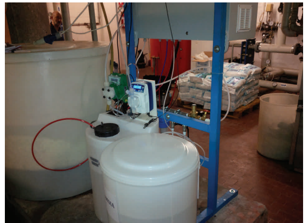
Dosing station with proportional and Redox pump
