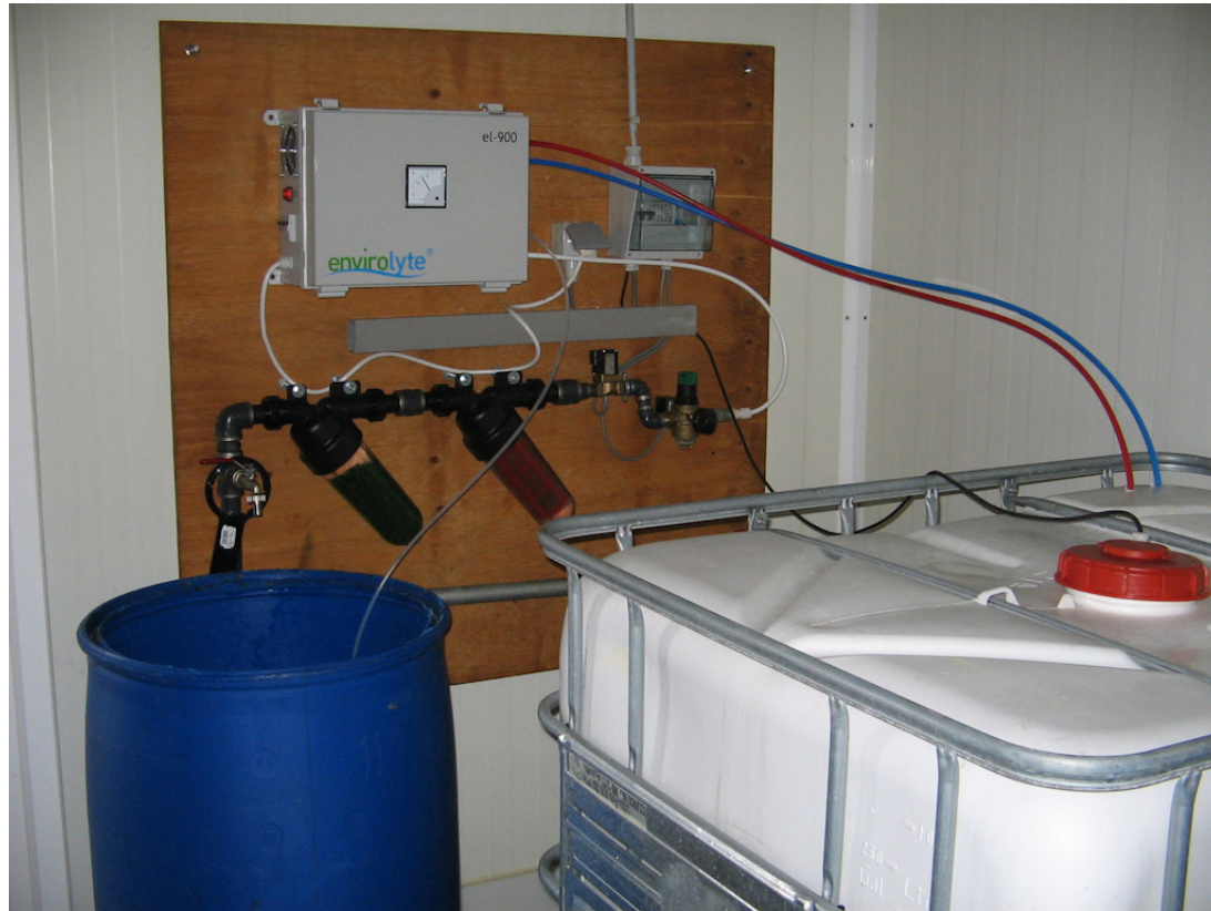
Automatization made by plumber
