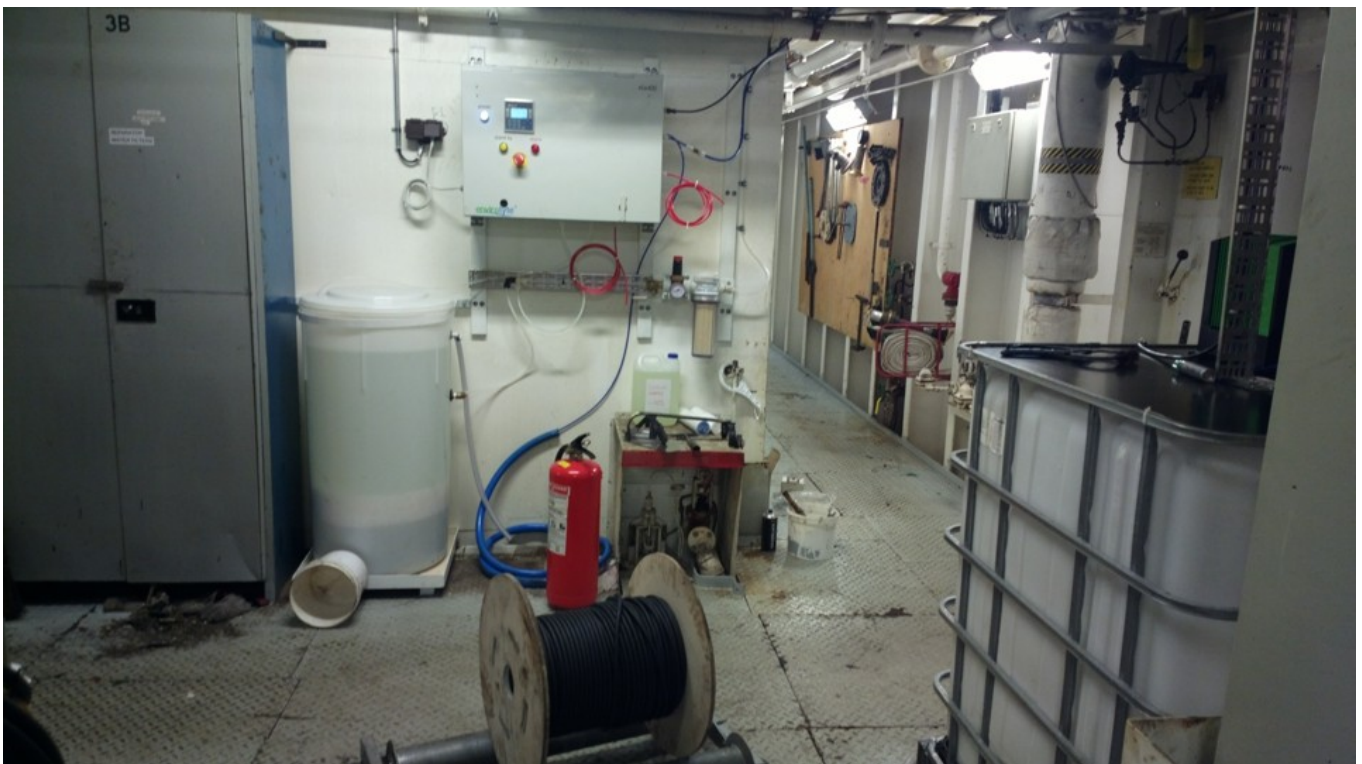
Envirolyte ELA-400 anolyte generator , brine tank, pressure control valve, water filter, pipes and fittings.
